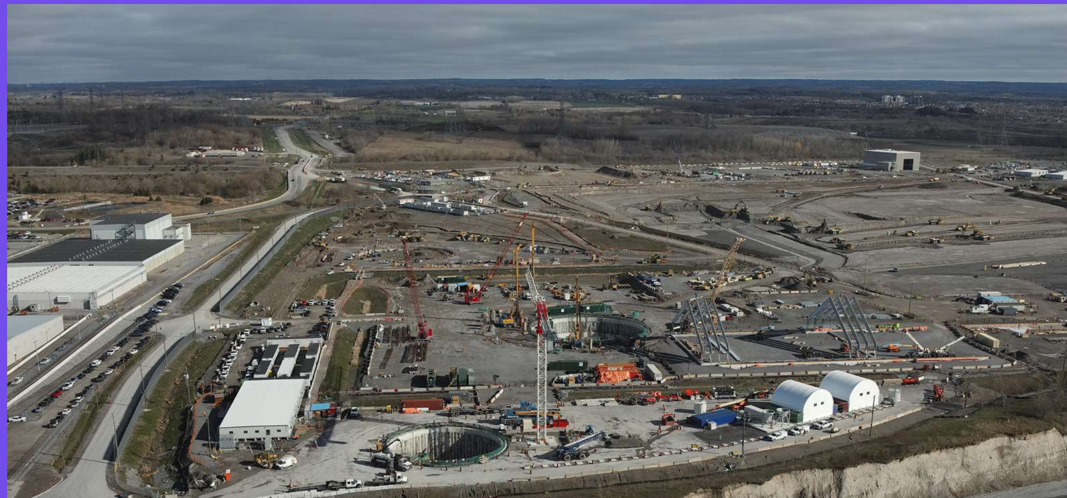
Construction of OPG's first of four BWRX300 SMRs at the Darlington, Ontario site. Source https://www.opg.com/wp-content/uploads/2025/05/DJI_20250430085020_0002_2732_crop.jpg
